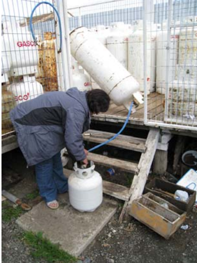
Jumper fill at Gasco bottle exchange retail location in Puerto Natales, Chile. Note inverted feeder tank.
