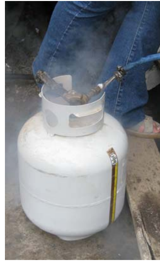
Note frost on the jumper line fitting. Liquid propane is very, very cold and will freeze your skin and tissue on contact.
