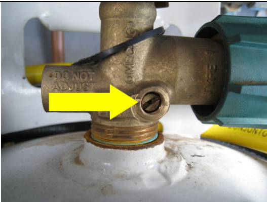
Bleeder valve on a QCC Type 1 output valve. The bleeder valve is the flat (slot) head screw.
