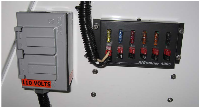
Garage 120 VAC outlets & 12VDC fused outlets
