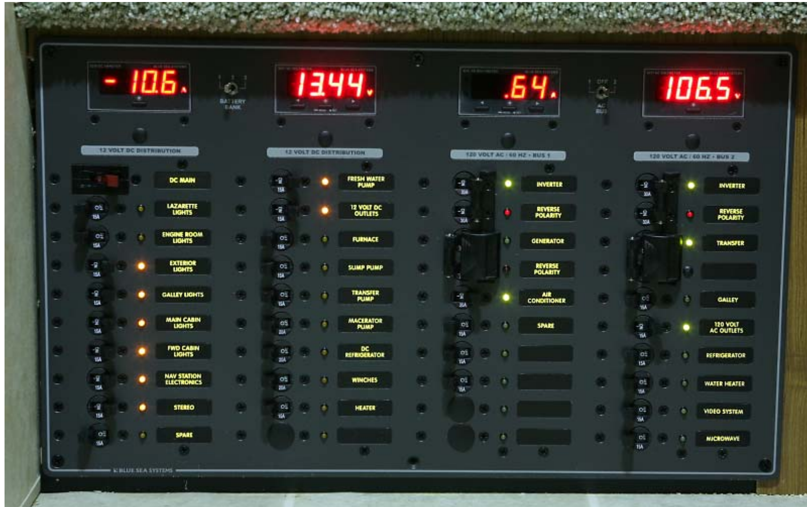
House 12 VDC / 120 VAC distribution panel with volt / amp / Hz meters
