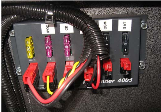
Center console 12VDC fused outlets
