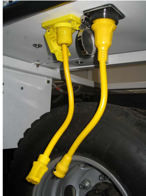
Shore and Guest AC power Input / Outlet connections with adapter cables. Left: guest power, Right: shore power. Input and/or output can be 120 or 220 VAC.
