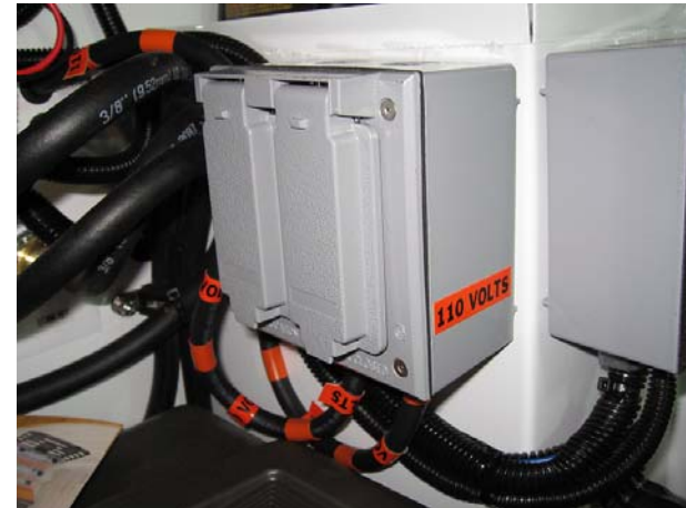
Shop 120VAC outlets
