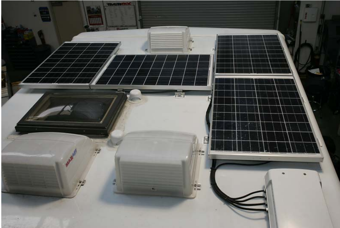
Solar panels and combiner
