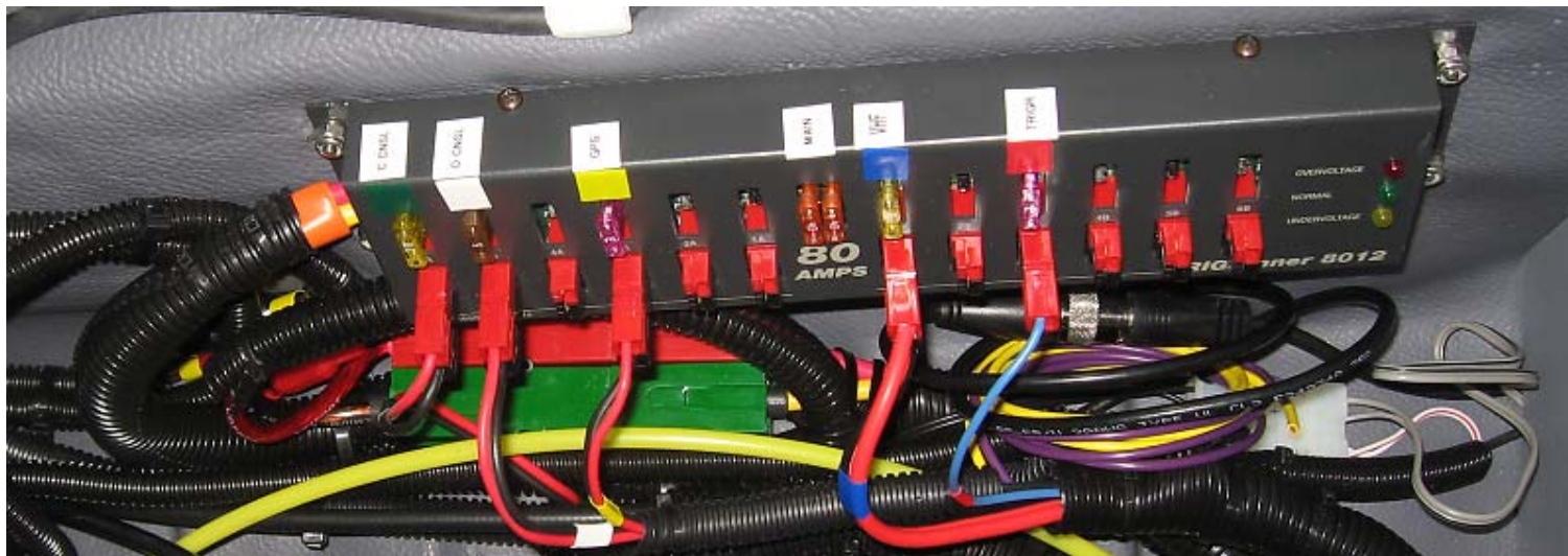
Cab 12VDC fused outlets / distribution
