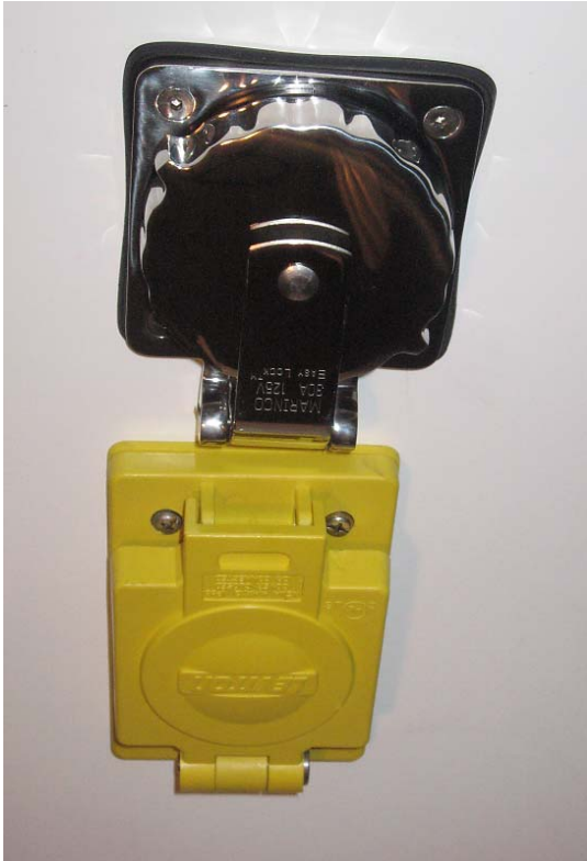
Shore and Guest AC power Input / Outlet connections. Top: shore power, Bottom: guest power. Input and/or output can be 120 or 220 VAC.
