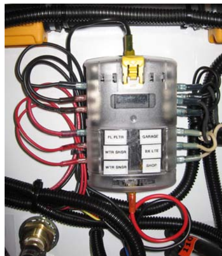
Shop 12 VDC Systems fuse block
