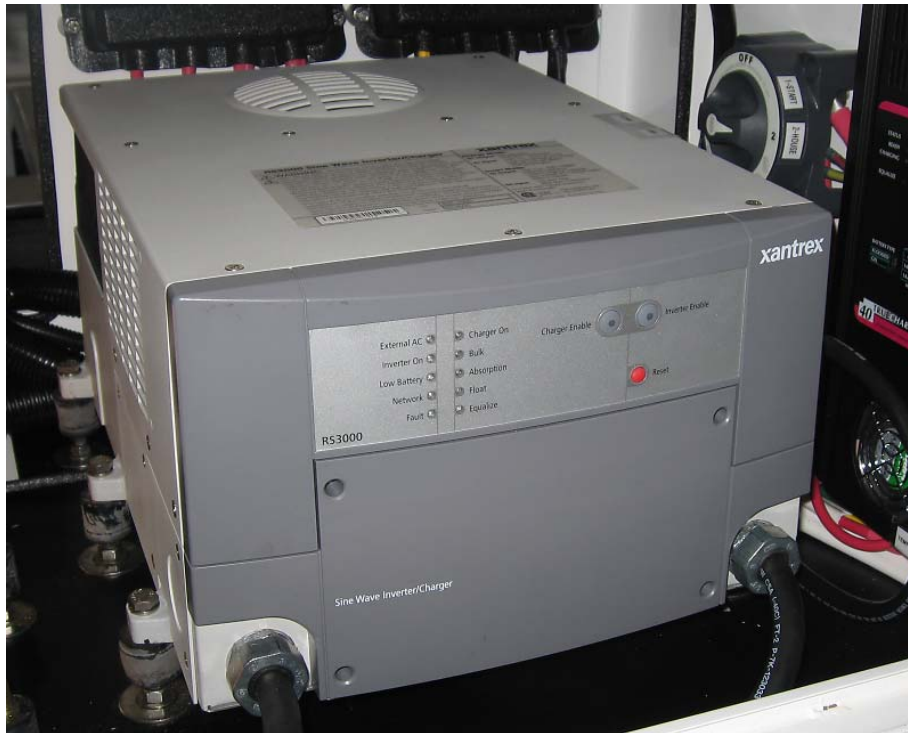
3,000 watt inverter / 3 stage charger
